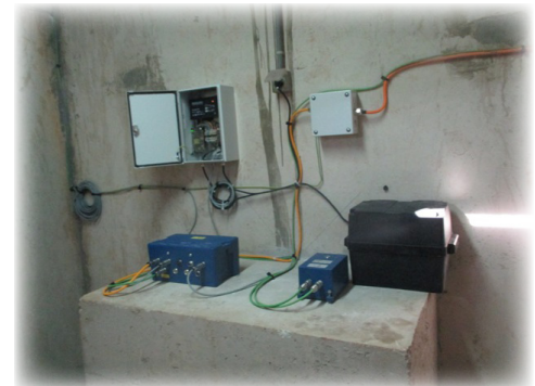
GeoSIG instruments at the seismic monitoring station at My Hassan 1st Dam.
