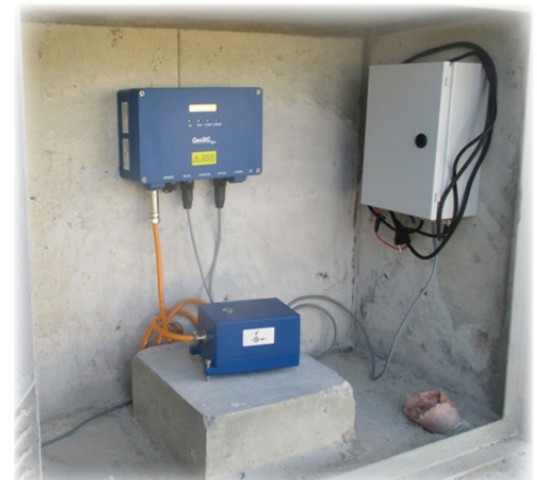
Martil Dam seismic monitoring station
