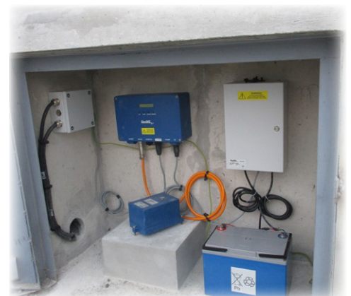
GeoSIG instruments at the seismic monitoring station at Dar Khrofa Dam.
