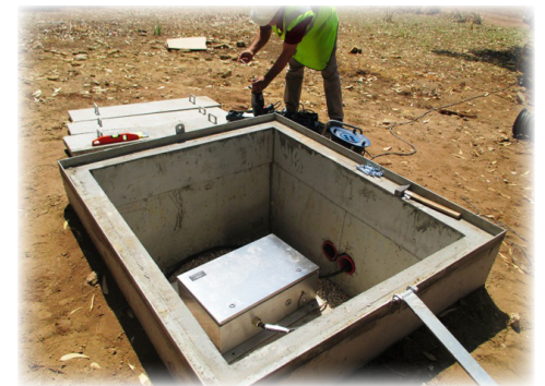
Rugged concrete vaults and heavy covering slabs protect installed instruments from the environment and vandalism.
